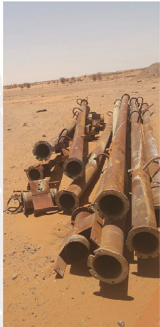
Corrosive pipe caused by bad quality water
