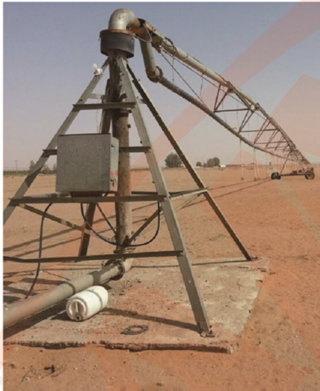
PE pipe under the steel pipe poor water application
